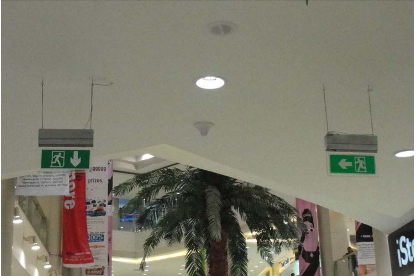
Signage's in Shopping Mall – Confusing exit signage - But here by putting two exit signage's creating a sign of confusion in the visitors mind that where to exit.
