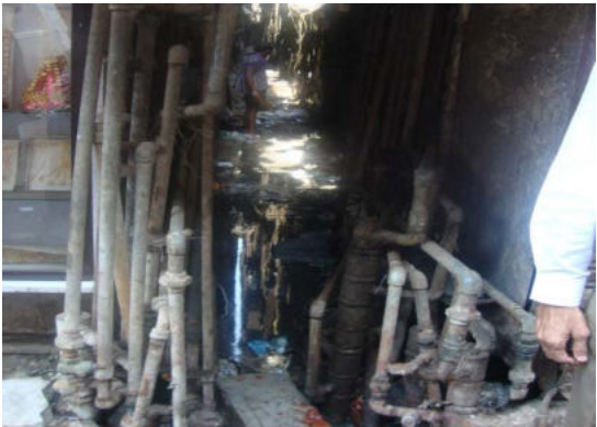
2. DRINKING WATER PIPES
