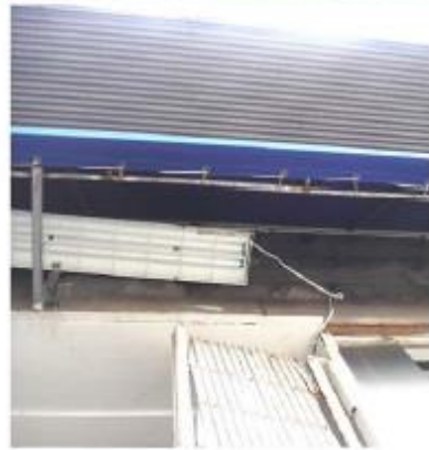
Site detail was little different from what was assumed- no ceiling was there to the canopy where we were about to drill the channels for the curtain
