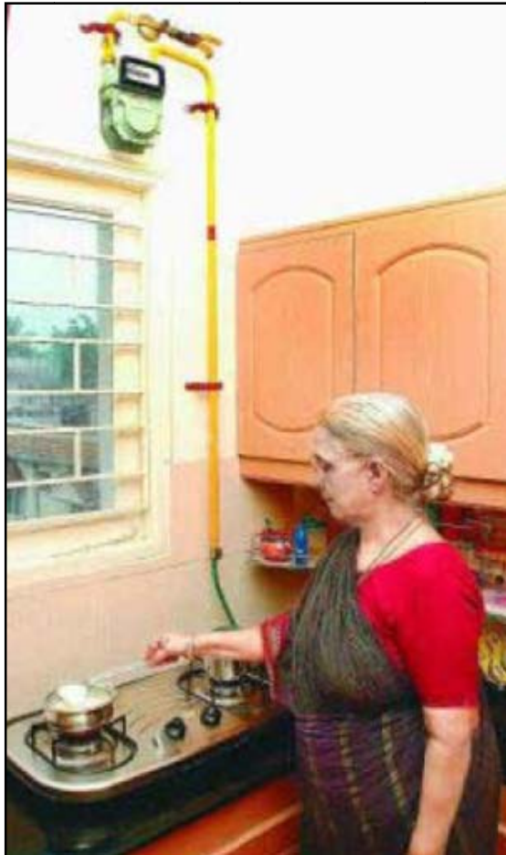
Image no. 1, Reticulated piping system
