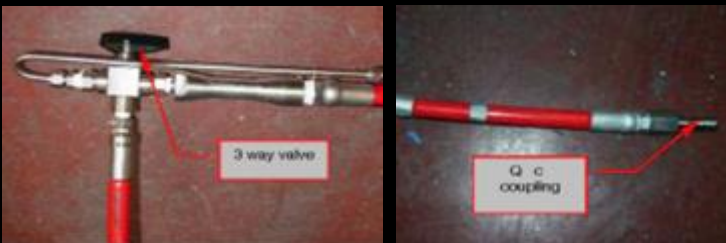
Three way valve hose
