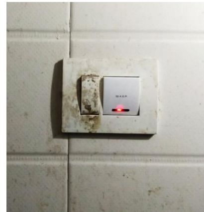
FIGURE-13 Switch of the wall concealed unit gets dirty in as it is located inside the bathroom.
