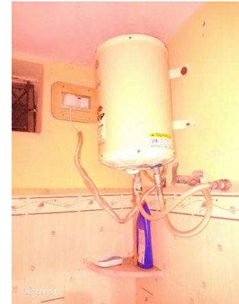
FIGURE-14 Water heater mounted inside the bathroom in the corner at with all pipes obstructing space of users to access.
