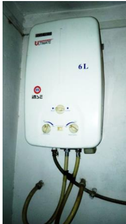
FIGURE-11 Water heater mounted at top corner of bathroom with almost not accessible to operator for people with shorter height.
