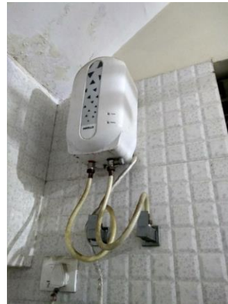
FIGURE-12 Water heater mounted inside the bathroom in the corner at high height of 8.5 feet.
