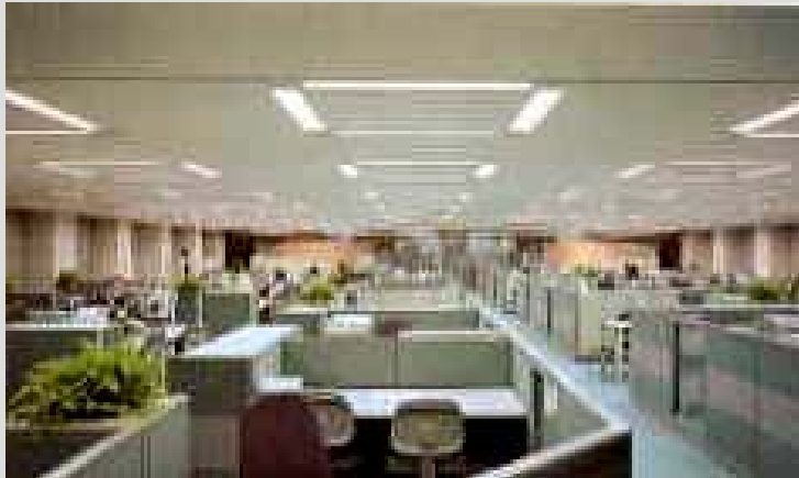
General purpose and task lighting in offices
