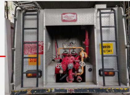
Water and foam two stage pump powered by diesel engine through PA coupling
