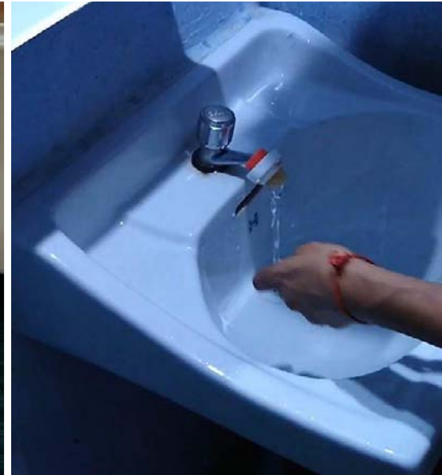
Fig: Washing face under Faucet (rural setting), For shorter durations of activities, users generally keep the faucet on.
