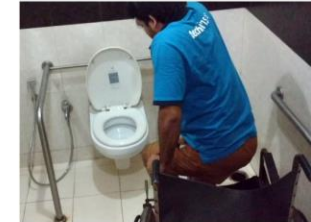
:Height of side panels and arm rest creates obstruction while shifting the patient from wheel chair to another transportation medium.
